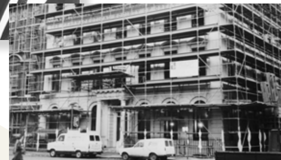
The Grade II listed building at 17 Bloomsbury Square underwent considerable renovations, courtesy of the Volkswagen Foundation. The Nash staircases with their wrought-iron balustrades and glass domed roofs were faithfully restored, the elaborate ceilings on the first floor were repainted using original 18th century pattern books, and exact replicas of the original crystal chandeliers were hung in the reception rooms.
